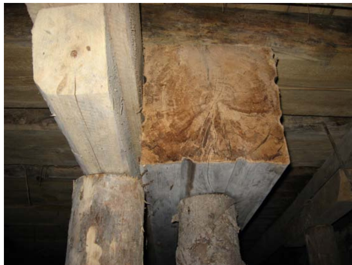
Figure 9: The main beam, an aged fruiting bodies of Serpula lacrymans and the timber, in the cross section, decayd by fungi.
