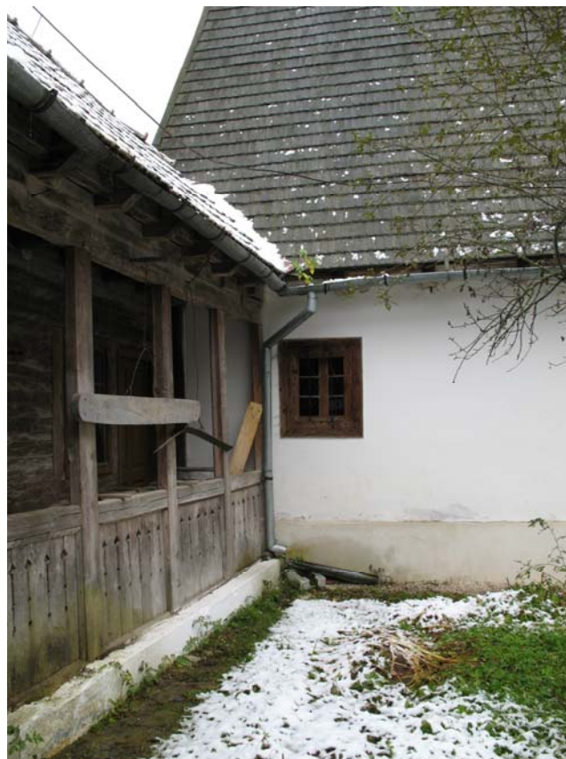
Figure 5: Rain-pipe flows damping the contiguous wall.
