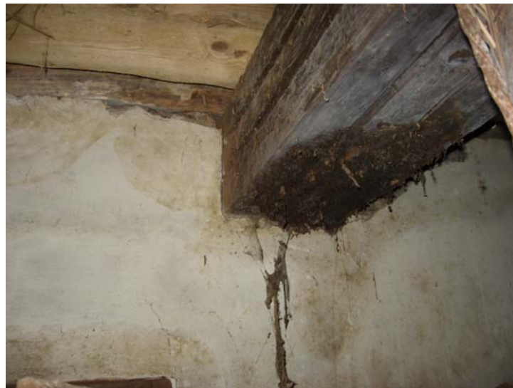
Figure 8: The main beam, an aged fruiting bodies of Serpula lacrymans and the timber, in the cross section, decayd by fungi.
